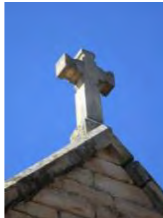
Plate 62. Evidence of re-mortaring between the sandstone blocks.
