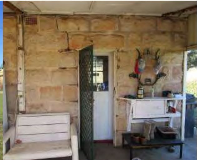
Plate 45. Evidence of cracking in sandstone wall of kitchen.
