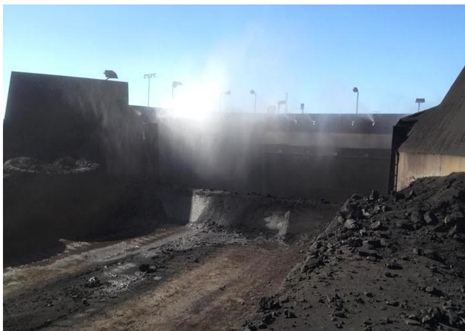
Figure 4: Sprays on ROM bin
