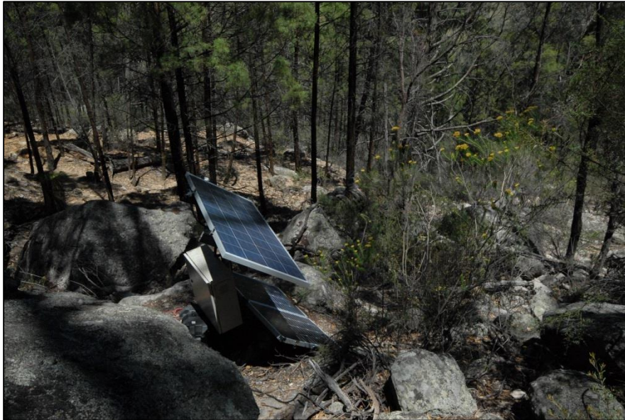
Figure 4.31 Supporting infrastructure for monitoring equipment, erected a short distance from WCP152.
