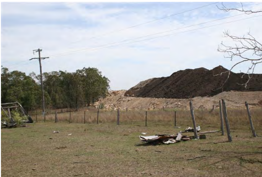
Figure 4 - Visual bund being constructed near old homestead. It will be important to shape the bund so that its surface profile is rounded and slightly irregular so that it is compatible with the surrounding landscape forms.
